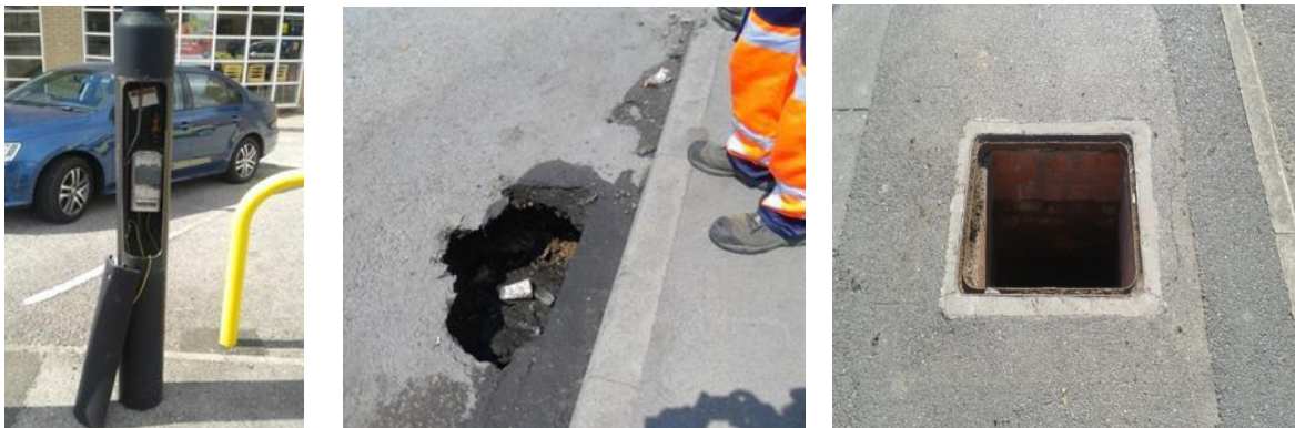
Lighting Column access cover Carriageway Collapse Missing Chamber Cover Removed exposing cables
